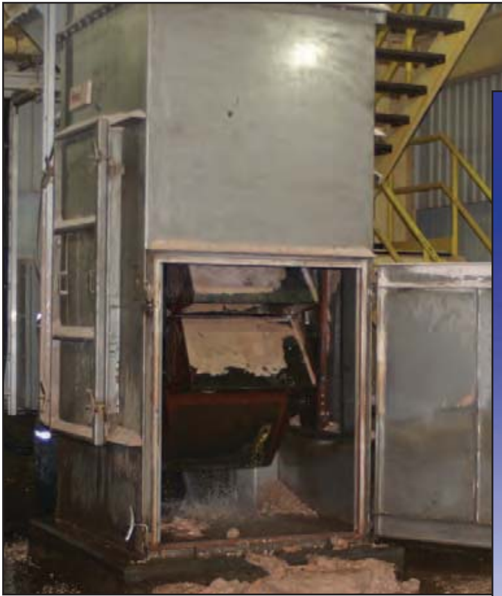
Large doors provide easy access for cleanout, inspection and maintenance.
